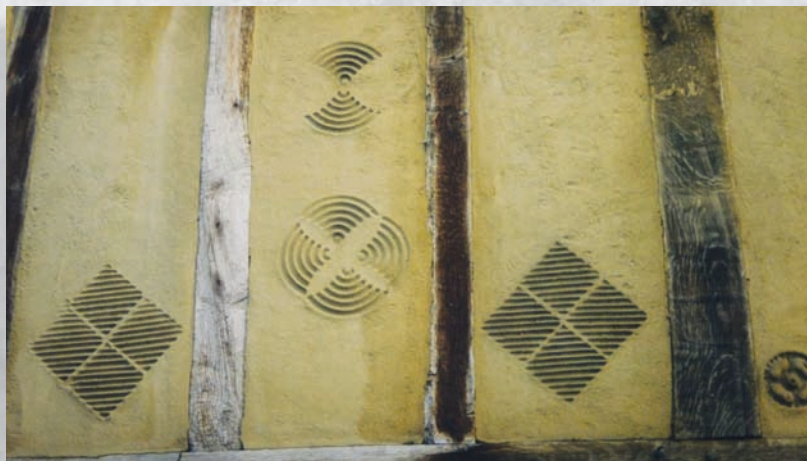
Below right: Pargetting with various "press rolls" on a timber-frame wall in Saffron Walden, Essex, England
